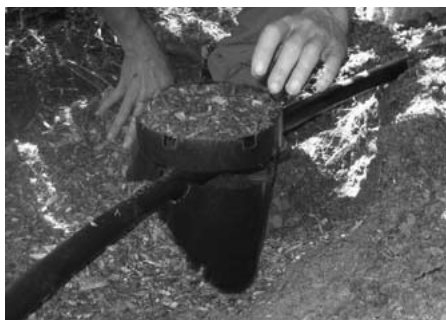
Outlet shield in mulch basin (5 gal pot).
