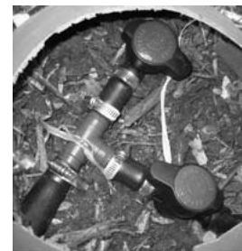
Zone valves in valve box made from a recycled plastic drum.
