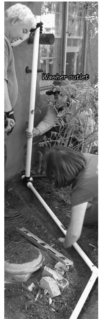
Leveling a Laundry to Landscape line buried 4" deep in a hard-freeze climate. This line ran fine all winter, even though the plumbing inside the house froze!
